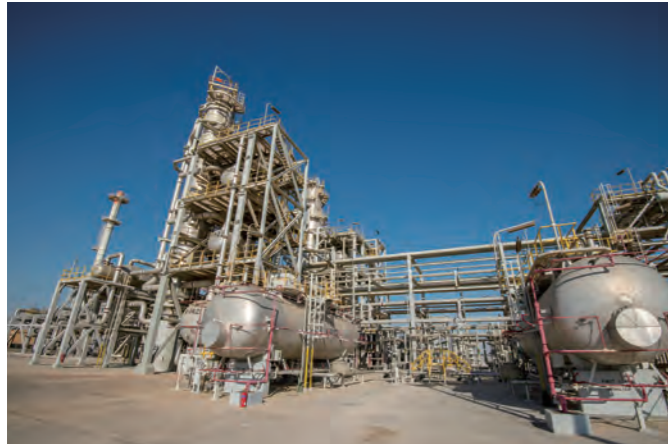
Abu Dhabi Onshore Concession production facilities
