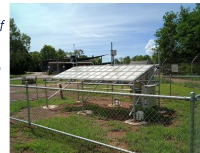
Artificial photosynthesis panels installed in Darwin, Australia
