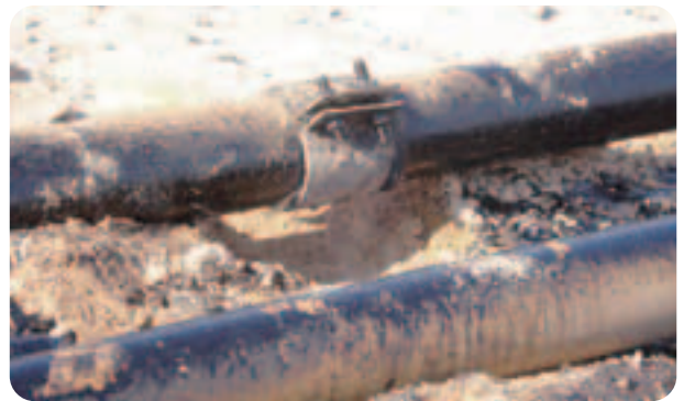
Pipeline requiring repair
