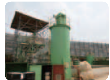
Drilling fluid treatment unit
