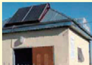
Solar-powered water-purification facility
