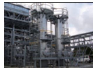
Hazardous substance removal equipment for gas condensate
