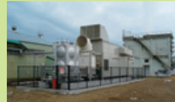
Natural gas cogeneration system
