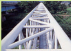
Natural gas pipeline operated by Teiseki Pipeline
