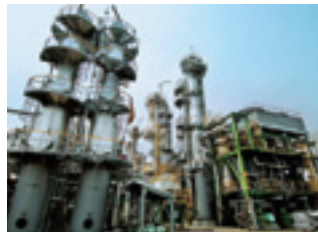
Gas-processing facility at Koshijihara Plant in Niigata Prefecture, Japan
