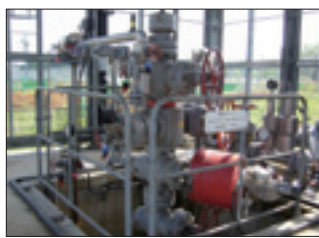
Injection/withdrawal well at Sekihara Gas Field
