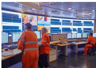
Control center inside the CPF
