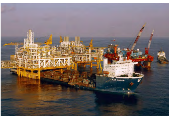
Offshore production facility, Bayu-Undan Gas-Condensate Field
