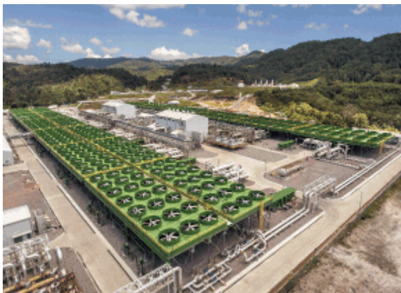
The third unit of Sarulla Geothermal IPP project
