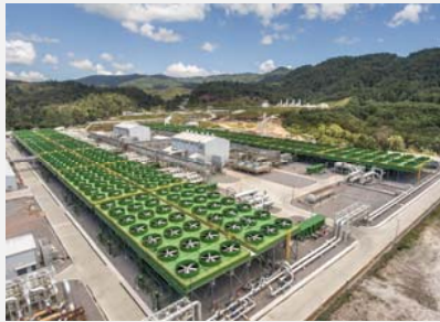
Sarulla Geothermal IPP Project
