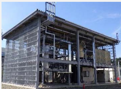
Methanation test facility
