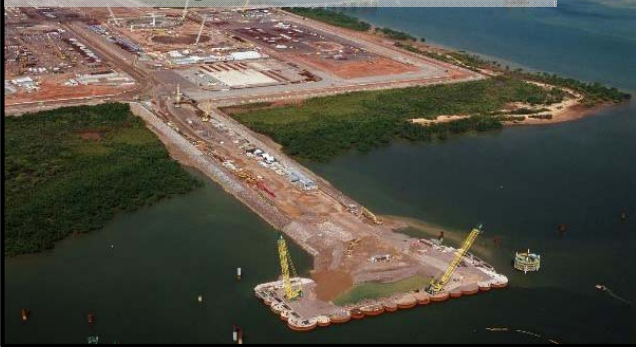
Module offloading facility of module for onshore LNG plant (Feb. 2014, in Darwin)
