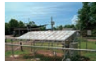
Artificial photosynthesis panels installed in Darwin, Australia
