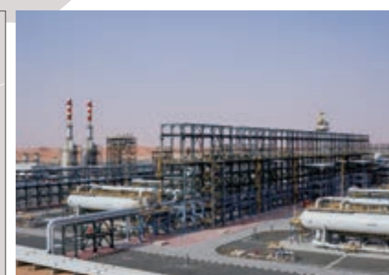
Oil processing facility
