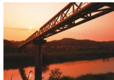
Natural gas pipeline crossing a river (Shibumi River, Niigata Prefecture)
