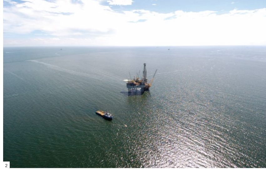
1: Booster station 2: Offshore platform during well drilling work
