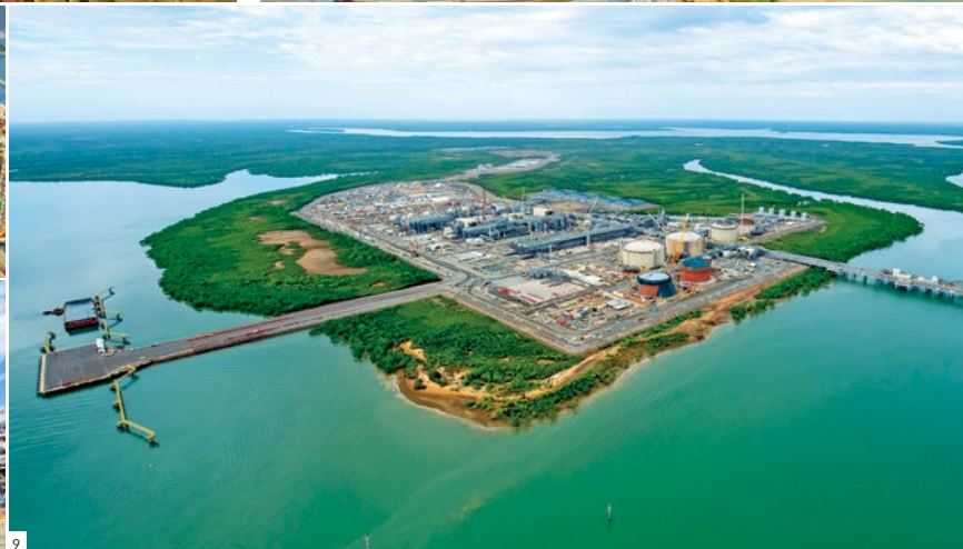
5: Gas export pipeline laying work 6: Onshore gas liquefaction plant under construction 7: Operations to install an FPSO's flare tower 8: Onshore liquefaction plant module installation operations 9: Onshore gas liquefaction plant
