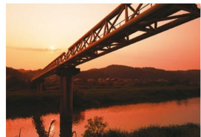
Natural gas pipeline crossing a river (Shibumi River, Niigata Prefecture)
