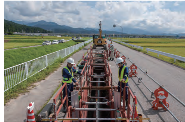
Laying pipeline underground with the Tateyama mountains in the background (Asahi, Toyama Prefecture)
