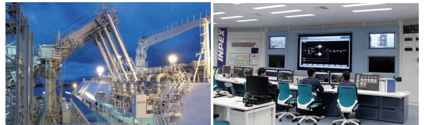
First receipt of LNG at the Naoetsu LNG Terminal LNG unloading operation (left); closely watched by the central control room (right)
