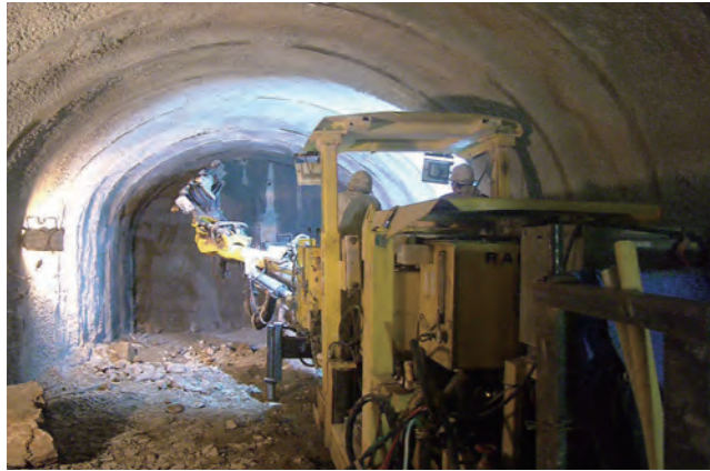
Five mountain tunnels drilled despite being hampered by hard bedrock and flooding (total length of approximately 12.6 kilometers)
