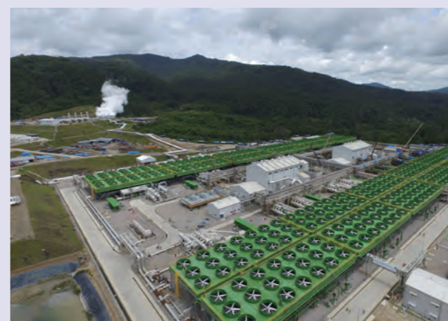
Operation started at Sarulla Geothermal Power Generation Plant (2017)
