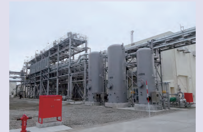
Low-pressure extraction equipment begins operation at Koshijihara Plant, Minami-Nagaoka Gas Field
